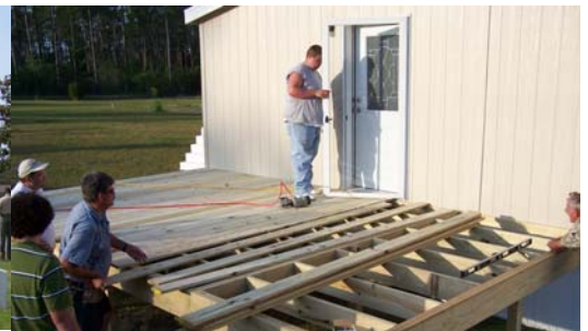
Sir Knights David Seymour, Tom Ross & Ed Creech begin construction on a deck/handicap ramp system
